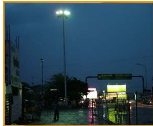
Fig: : High Mast Light – Integrated Bus Stand
