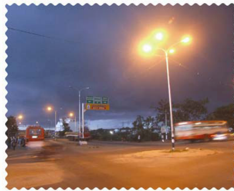
FIG: HighMask Street Light – Koodal Nagar
