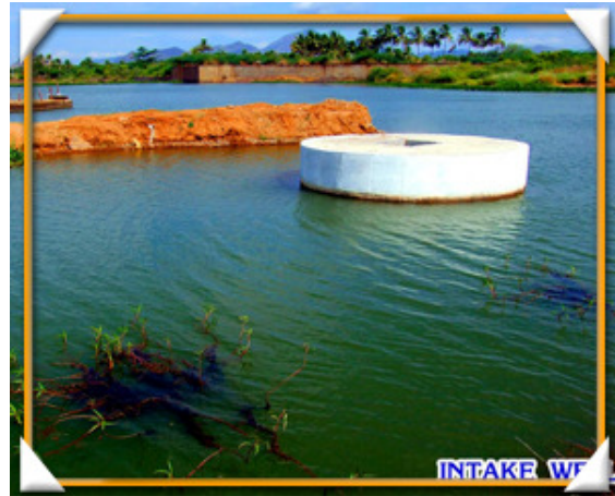
Fig: Intake well
